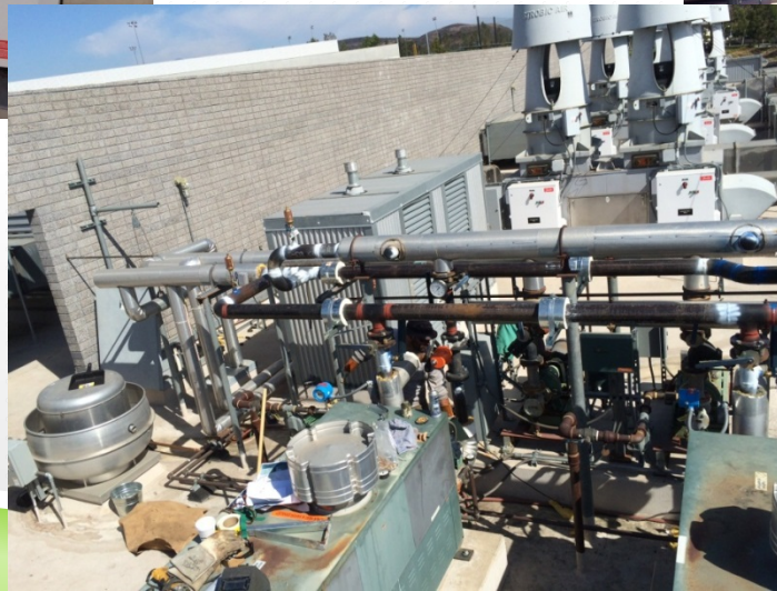
Controller, VFD Panel and Boiler Piping
