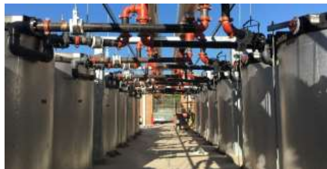
Figure 9. Cooling Tanks for Central Plant
