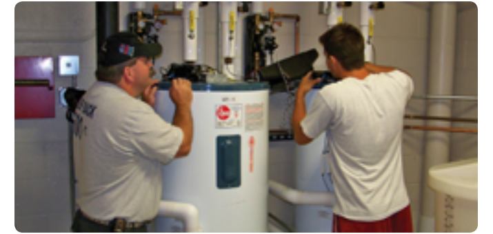
St. Clair County Community College students use data loggers to measure and analyze water temperatures as part of the new Siemens solar-powered hot water system in the college's Acheson Technology Center.
