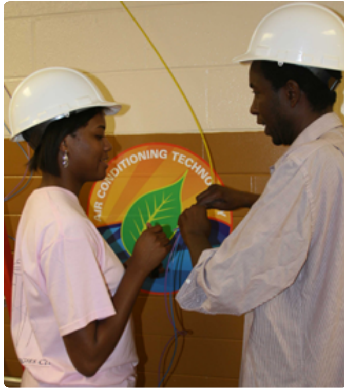
GPTC students install a communications network to track building conditions as a required, graded component of their course work. Both students have since graduated and are project managers at two building control companies in the region.
