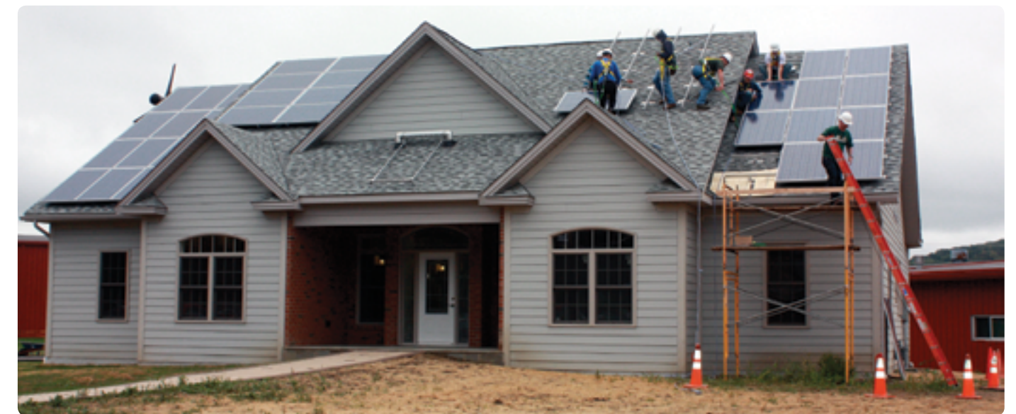
Students help to install solar panels atop Alfred State's net-zero model home.
