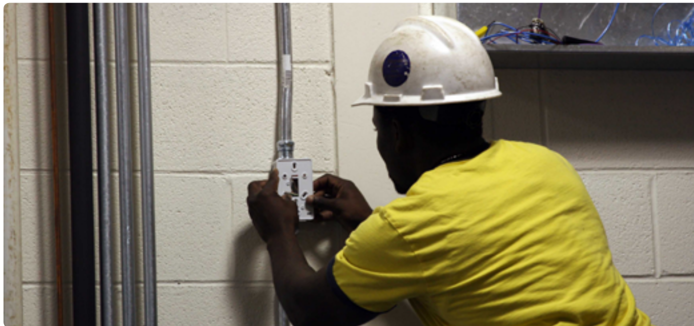
A building automation student mounts a sensor in GPTC's Green Technologies Academy.
