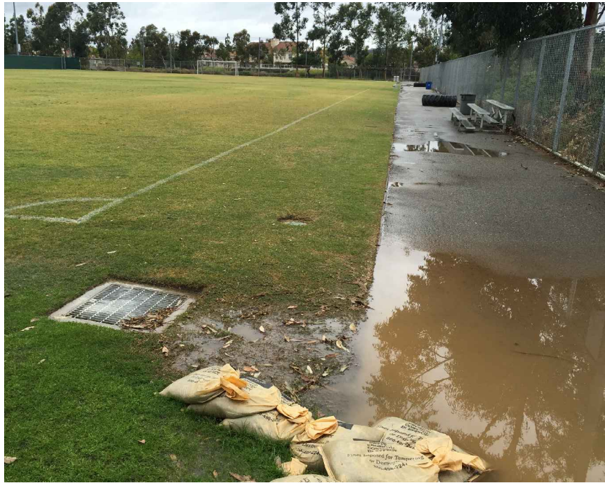
INLET ON SOCCER FIELD (FLOODING OBSERVED)
