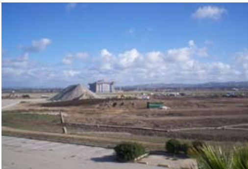
The Orange County Sheriff's Regional Training Academy site will be ready for foundations soon.
