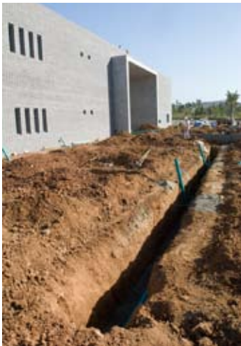
The Library/Resource Center's construction has moved ahead quickly since breaking ground in January 2005.
