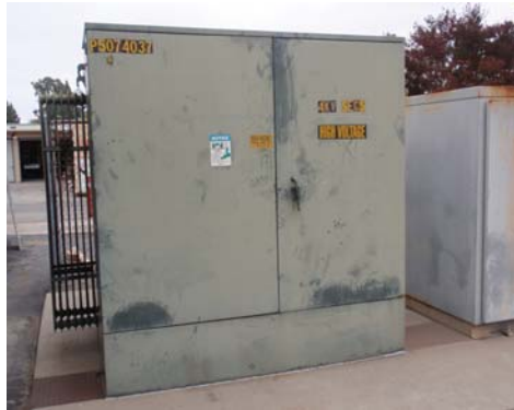
Typical Pad Mount Transformers
