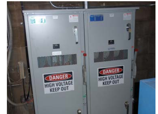
Typical 5-KV Air Switches
