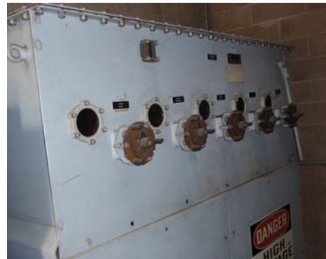
Typical 15KV Selector Switch in Building
