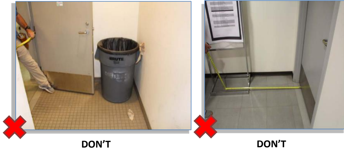
Trash receptacle and display rack obstructions located within required door clearances.
