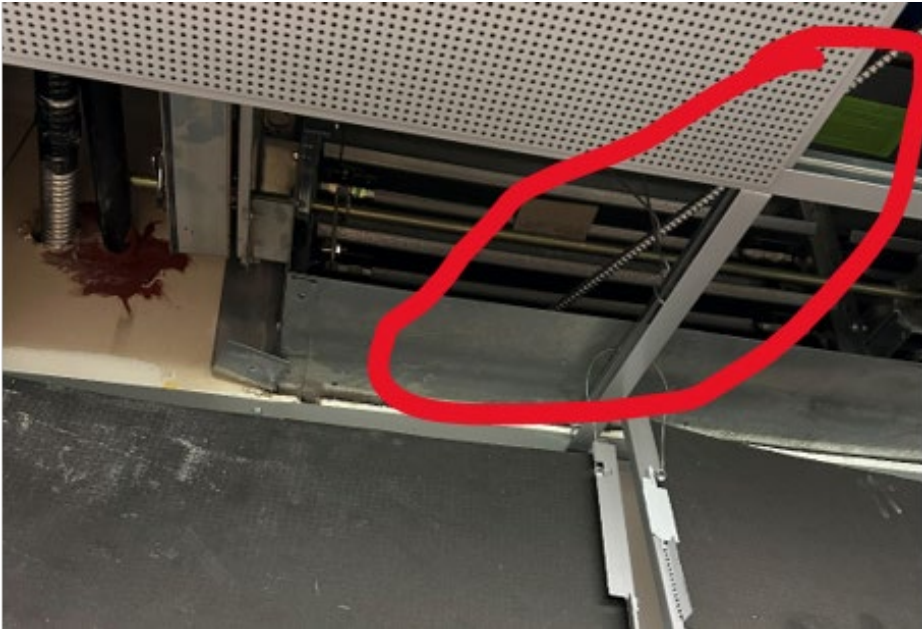
Example: flex conduit should not go through fire damper
